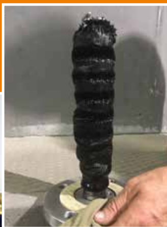
Ferro Cleaner magnet after 1 year of operation
